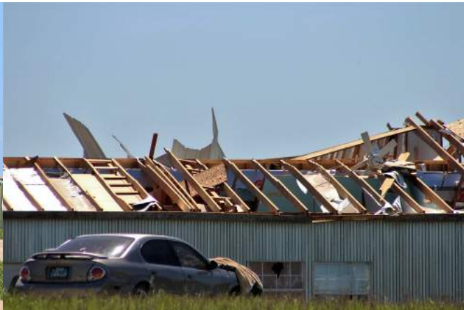
The roof of the Tapia home on Smith Road ripped off.
