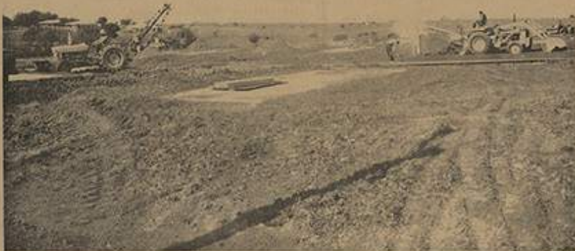
TWENTY-ACRE Mobile Home Park presently under construction is scheduled to be open in July, developers have announced. Work is progressing with concrete slabs, patios, service building, streets, and other phases of the project. General Contracting Company of Garland is in charge of the construction.
