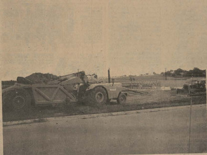
GROUNDWORK for a new 100-unit apartment complex was started within the past week, when heavy machinery was moved in to level the area just west of the expressway. The complex will be housed in 14 buildings, with completion date set in nine months. New White A to store building is in background.
