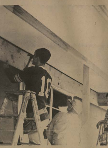
New home continues to grow as shown here on the Hill Stamborough home in North Howe, Contractor for this project is Bill Mayo (Photo by L. L. Lisker)
